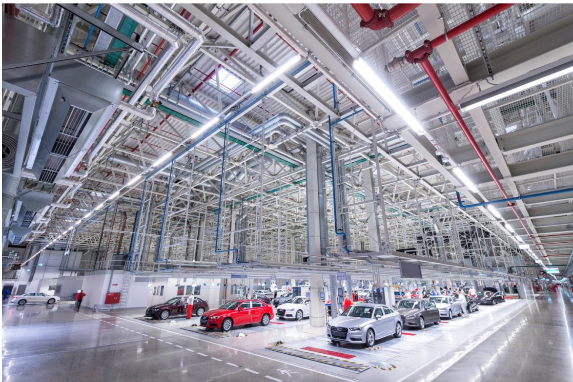
Fig. 2: In the assembly bays, more than 140 kilometres of the TECTON continuous-row lighting system were installed.
